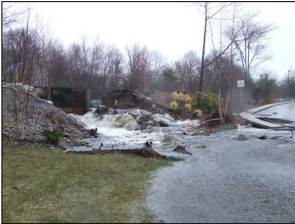
Failure of privately owned dam in Canton Photo Credit Robert S. Stephens, PE
